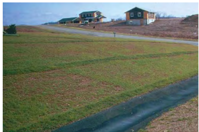
Figure 6.13. Adding single strips of sod to seed establishments on sloped sites is a highly effective means of reducing soil erosion potential.
