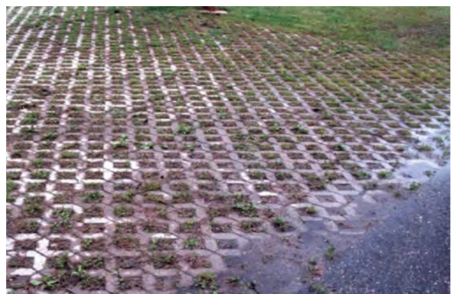
Figure 9.9. Compost can be used as partial growth and filtering medium in pervious pavement.
