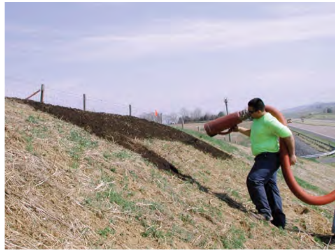
Figure 9.10. Compost applied pneumatically to steep slopes adjacent to highway to establish medium for erosion controlling and hillside stabilizing vegetation. Photo courtesy of Greg Evanylo.
