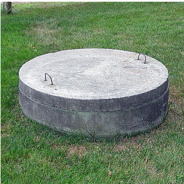
Figure 1b. A bored well with a tightly fitted concrete cap. Source: Bryan Swistock, Penn State University.
