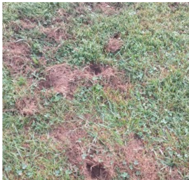
Figure 4. Animals digging for grubs near the surface of this lawn have caused this damage.
